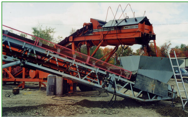
The CROSS-FIRE unit feeding a stacker conveyor, returning cleaned soil to the excavation. As much as 45 tons of contaminated soil can be cleaned in an hour.
